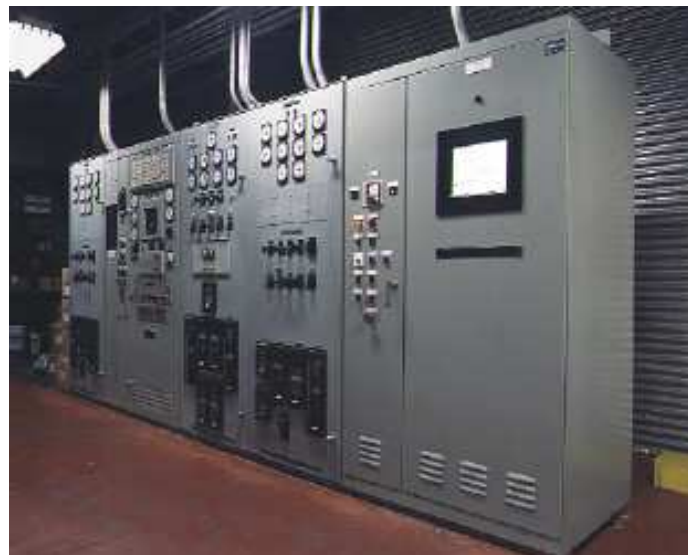
Replacement controls for one GE LM2500 gen set in LNG plant power service.
