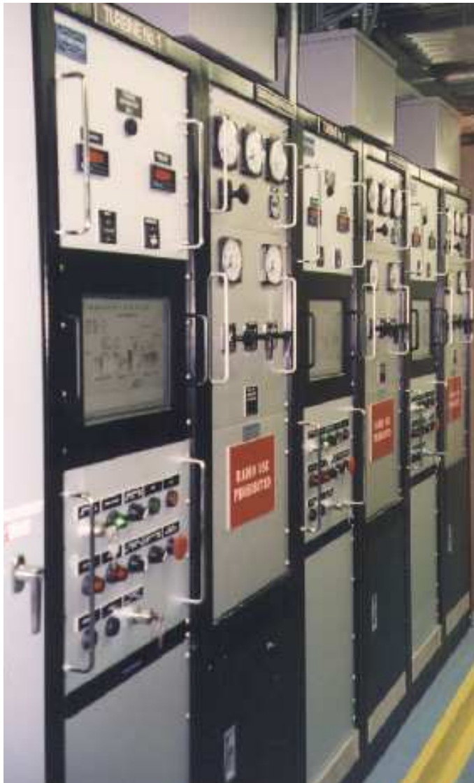
Replacement controls for two Allison 501K gen sets in emergency backup power service.
