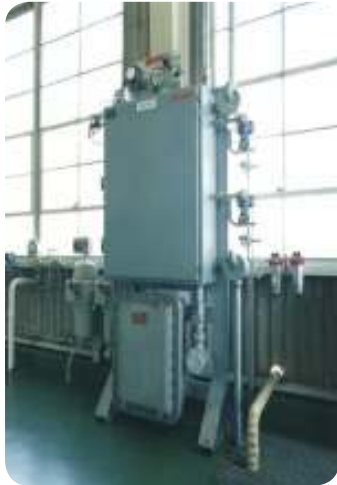
One of six engine/compressor local unit control panels.
