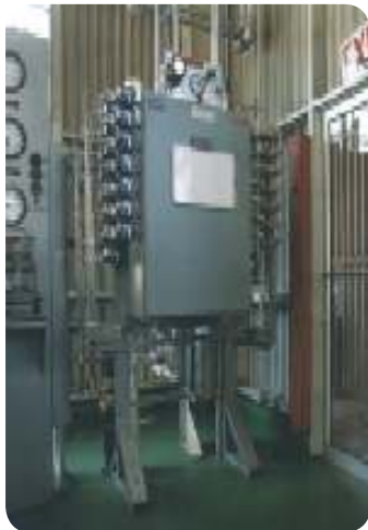
Torque control interface panel for a gas pipeline station.
