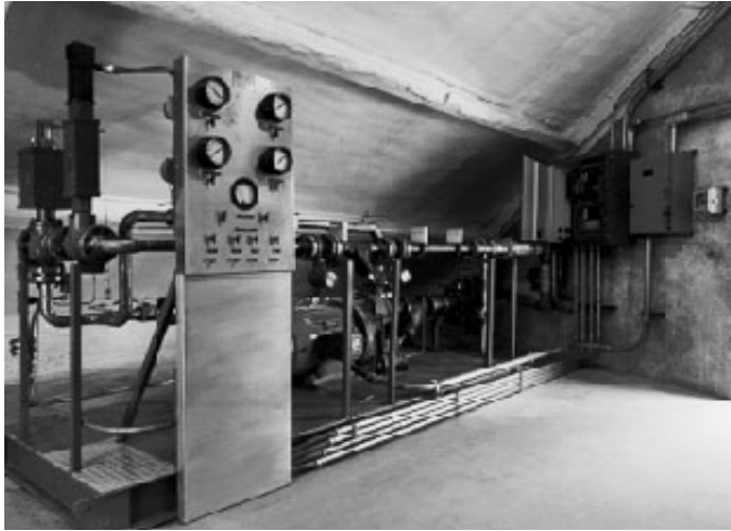
Installation of a water injection pump and flow control skid for a Frame 7 gas turbine gen set in utility service.
