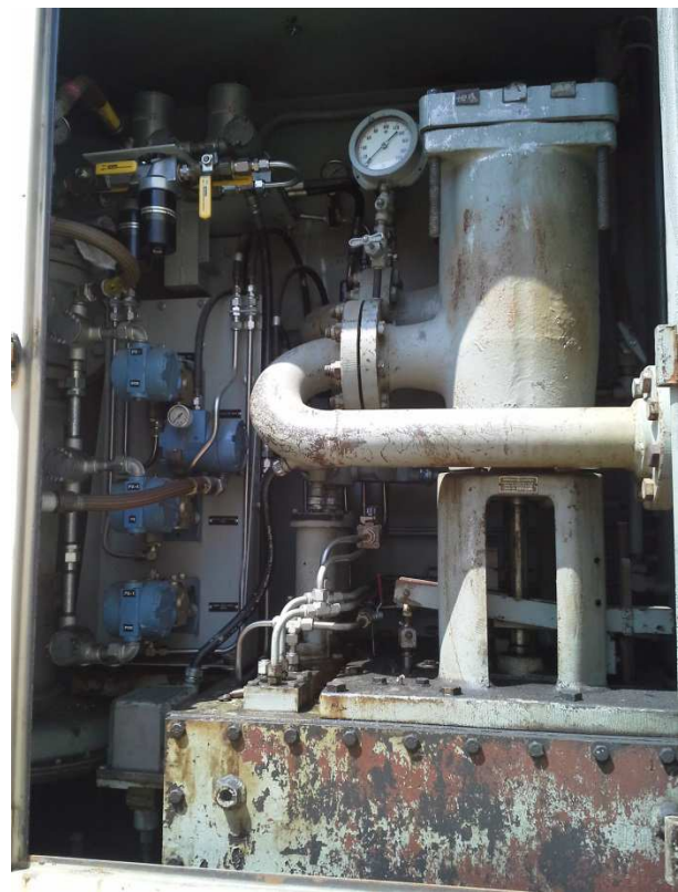
Figure 1 - Fuel Gas Cabinet prior to Single Fuel Control Valve Retrofit
