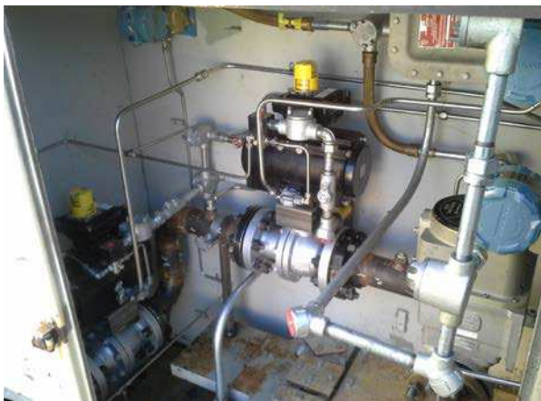
Figure 4 - Fuel Gas Cabinet after a retrofit to Single Fuel Control Valve Control System
