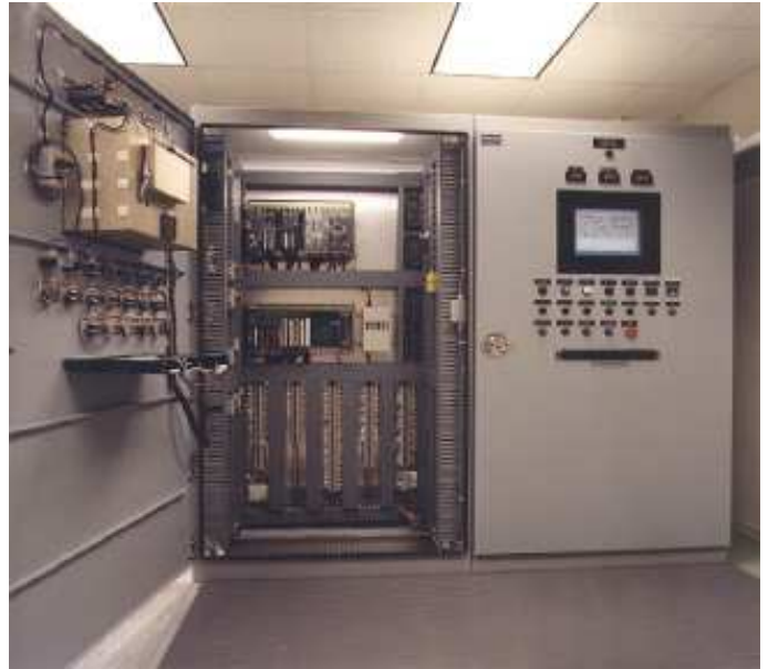
Replacement controls for two Allison 501K compressor sets in pipeline service
